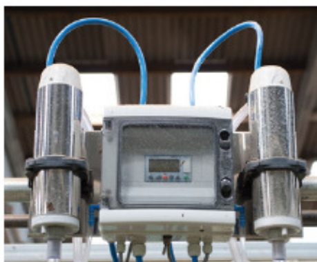
Above: a pair of pressure vessels and controller mounted in a swingover parlour
